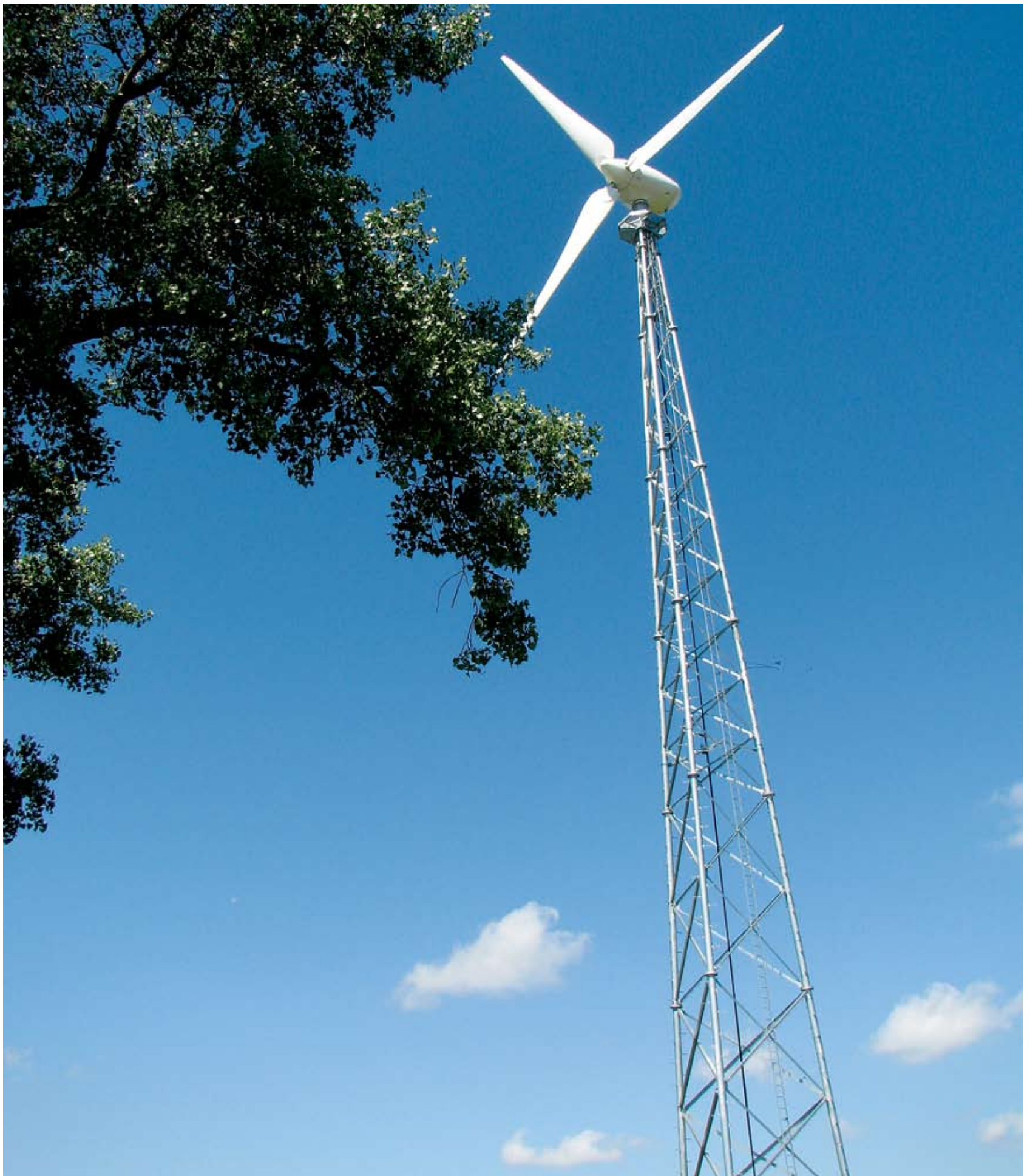
The wind turbine supplies the farm's electricity.
